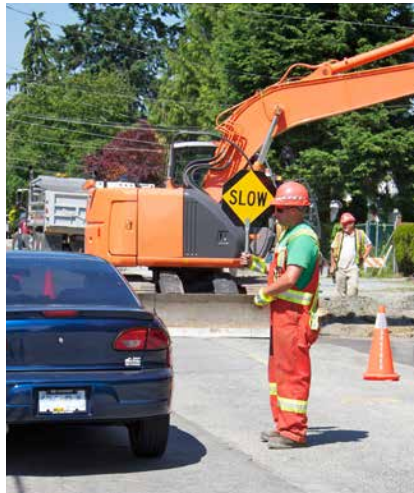
Each roadside worksite is different – be aware of the hazards.
